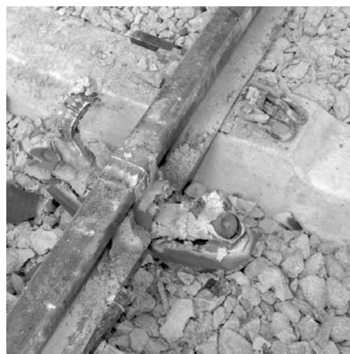
Figure 2 Gaps between the rails joined together tightly when the iron cooled.
